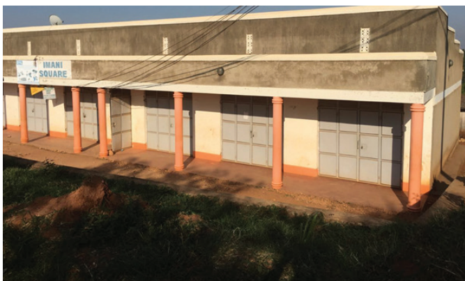
Photo 3: The dilapidated building that houses the Kyegegwa Chief Magistrate Court Premises. On the day we visited goats were roaming around the court premises.
