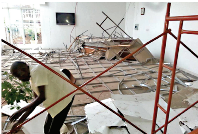
Photo 1: Ceiling that collapsed in Twed Towers (the building that houses the Constitutional, the Criminal and the Land Divisions of the High Court).
